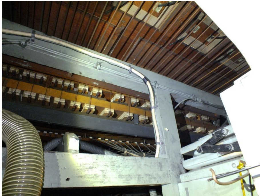
Underside of Grand Orgue soundboard, showing 1913 Lewis & Co. underaction acting on the jeux de combinaison pallets, and cross-tracking linking these to the jeux de fonds pallets
