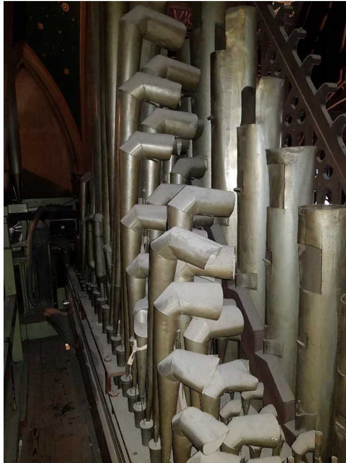
1893 Cavaillé-Coll Tuba mirabilis 8' and Clairon 4' on 1913 Lewis & Co. soundboard immediately behind façade
