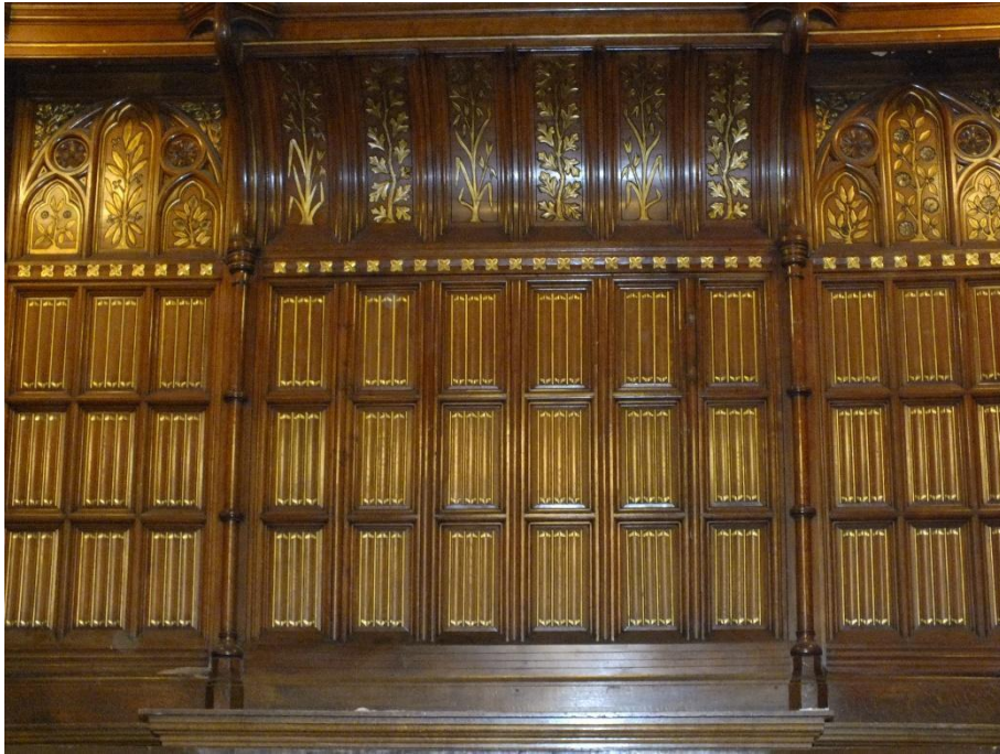
Lowest 12 of the centre panels are non-original
