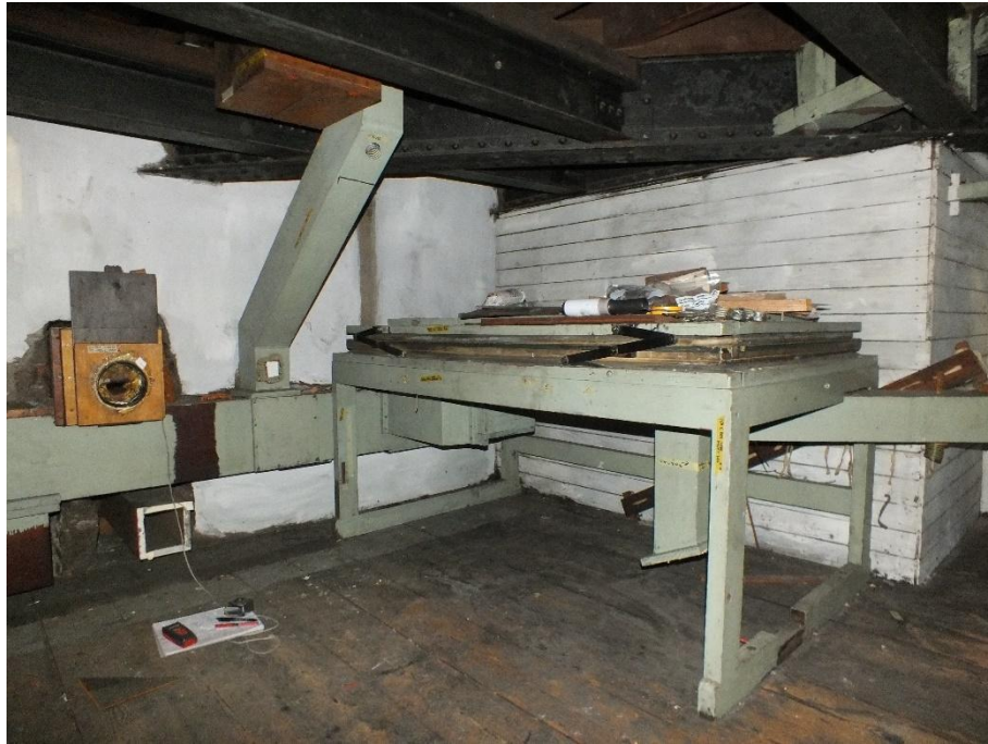
C side trunking and reservoir
