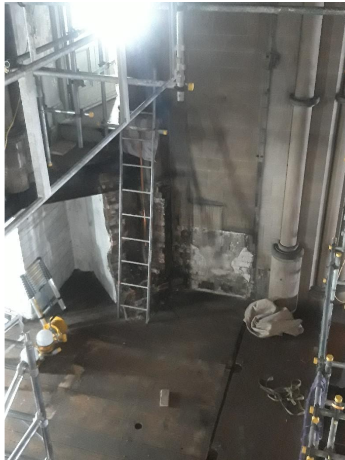
Tide mark and demolished brick support for bass side staircase
