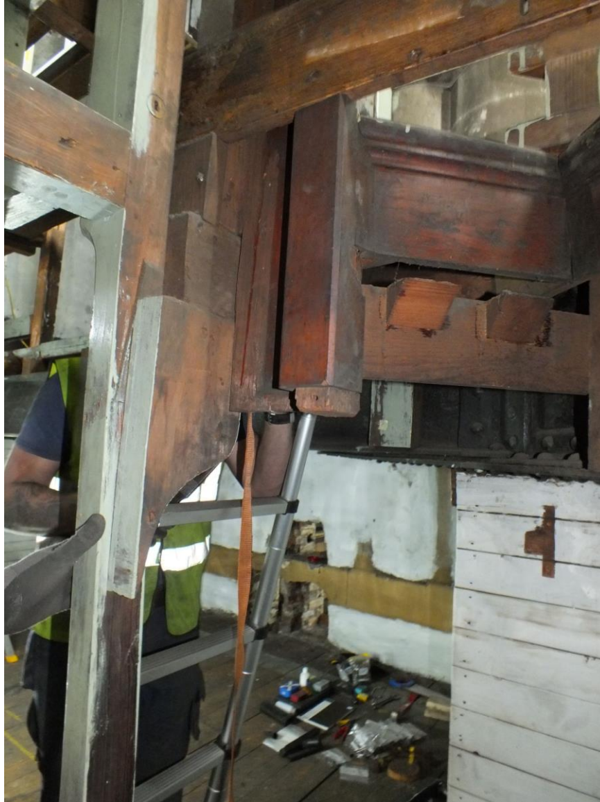
Part of the supporting structure of the staircase bracketed onto the Cavallé-Coll building frame visible on the left
